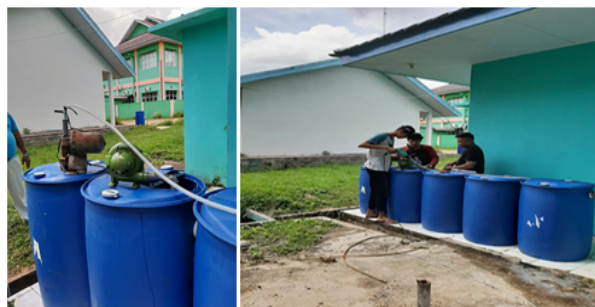
Figure 1. Blower and Water Pump
